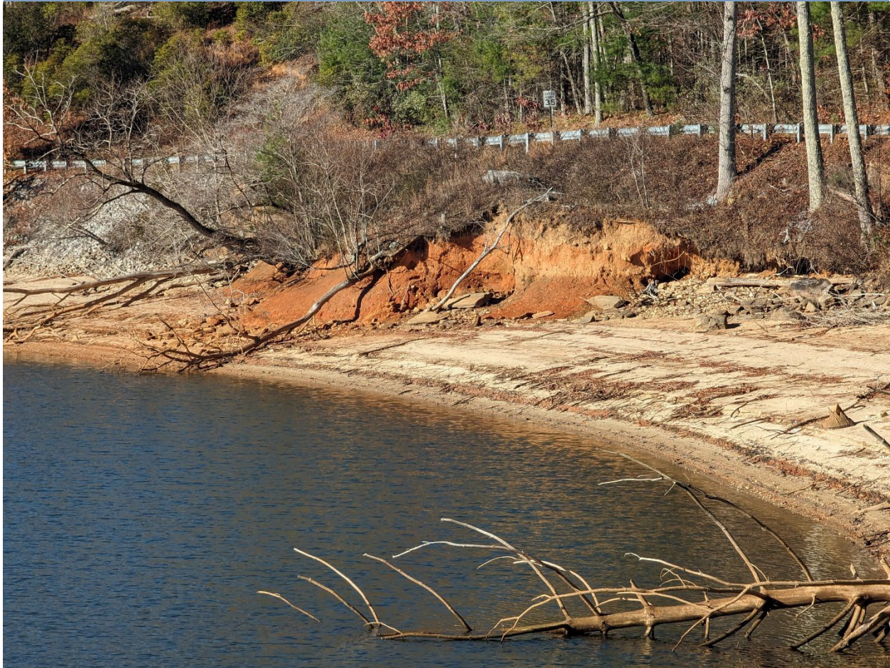
Figure 9. Eroding and slumping bank along the lake shoreline. There are not many areas like this on the lake, due to the large amount of bedrock along the shoreline. However, these are potential problem areas where wake and wave action can increase sediment load to the lake.
