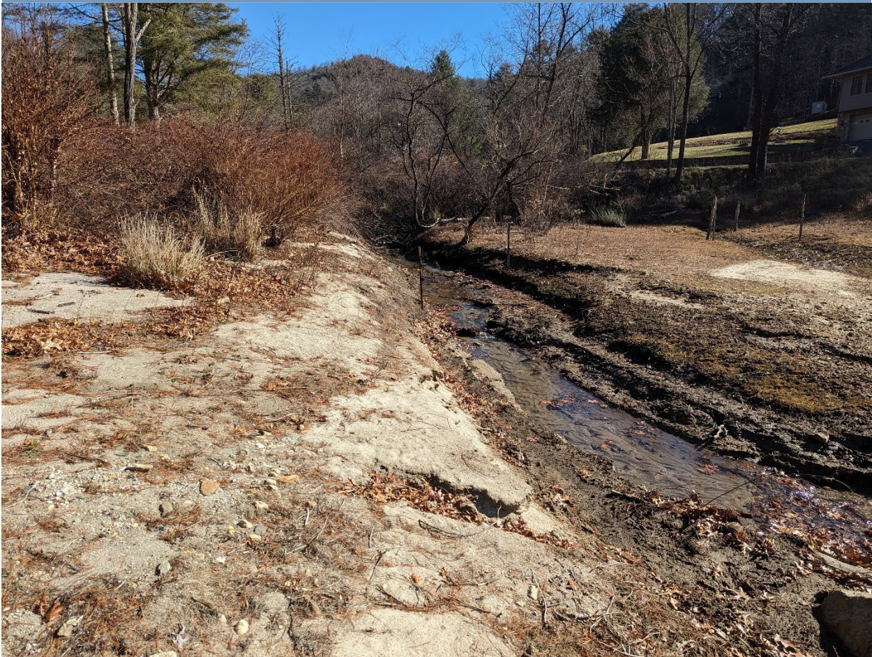
Figure 10. Delta formation at the confluence of Glenville Creek with the lake. This area appears to be relatively healthy wetland transition from stream to lake, though increased deposition and aggradation could fill it in over time.
